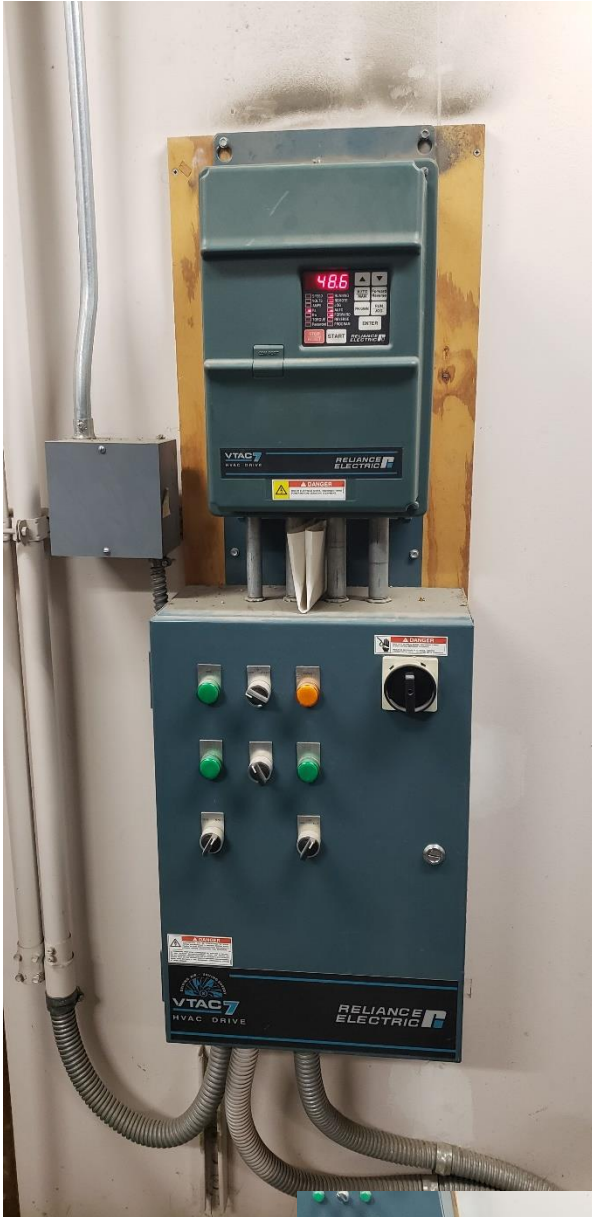
V-Tech Cooling Tower Pump Drive
