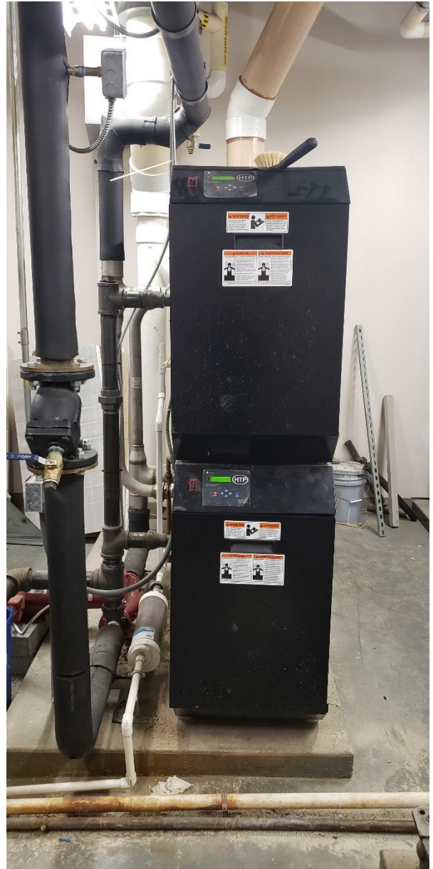
Condensing Boiler (Modcom 1440)
