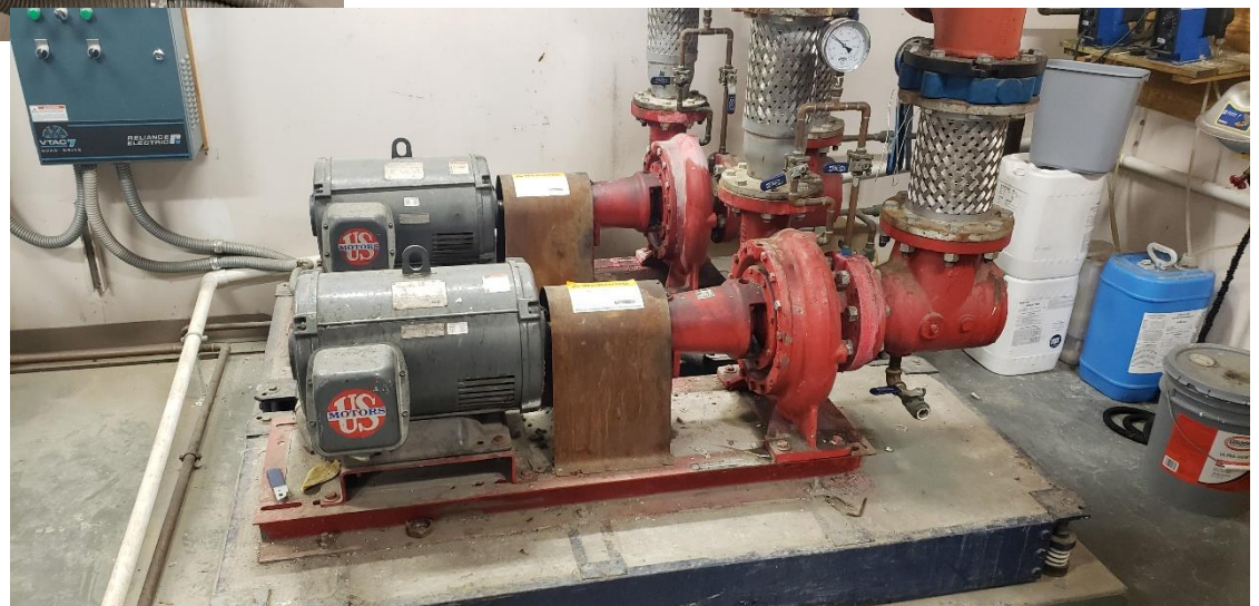
25-Horsepower Cooling Tower Pumps
