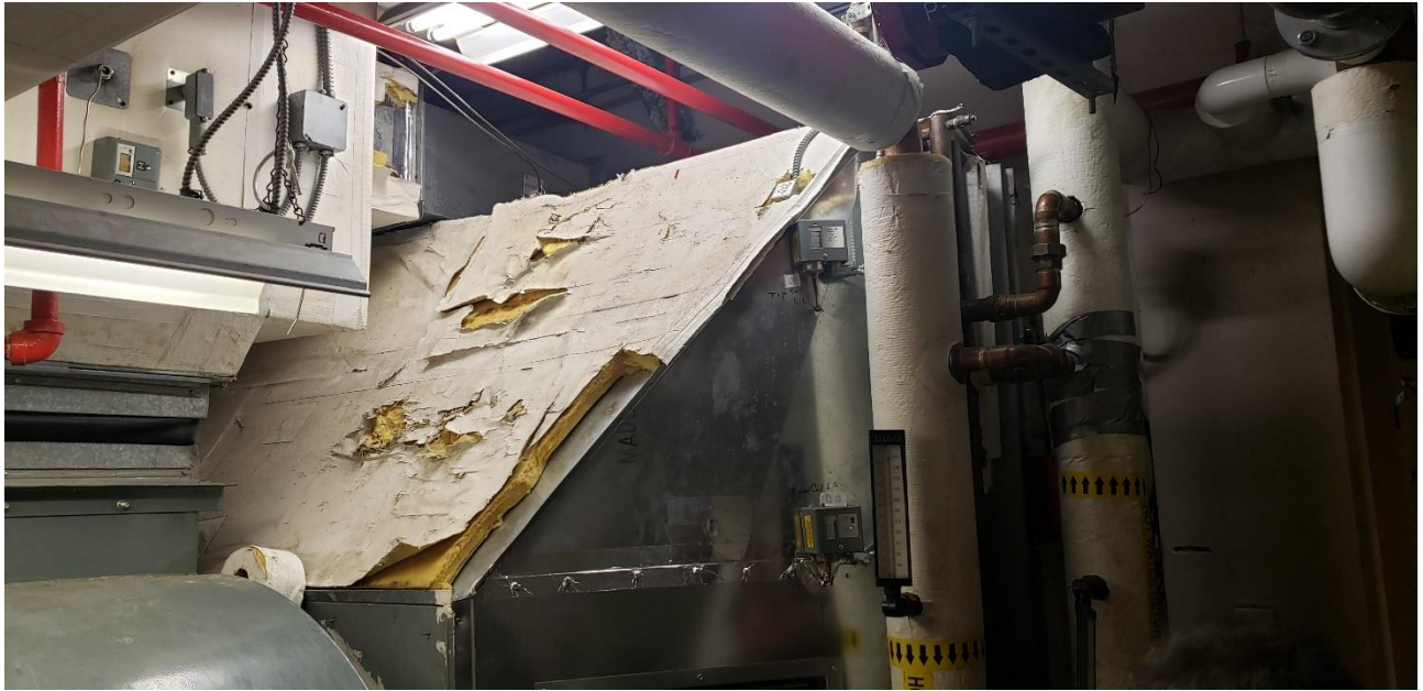
Ventilation Supply Fan S-1 with Outside Air Intake Ductwork
